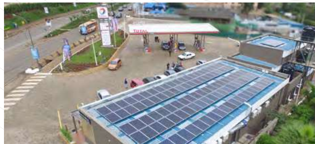
Solar panels at the Total Kenya Service Station in Gigiri, Nairobi
