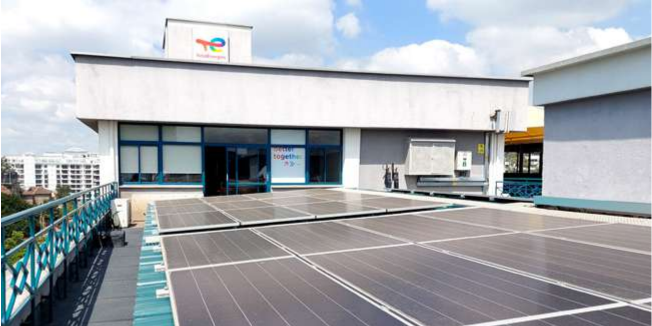
Solar panels installed at our Head office
