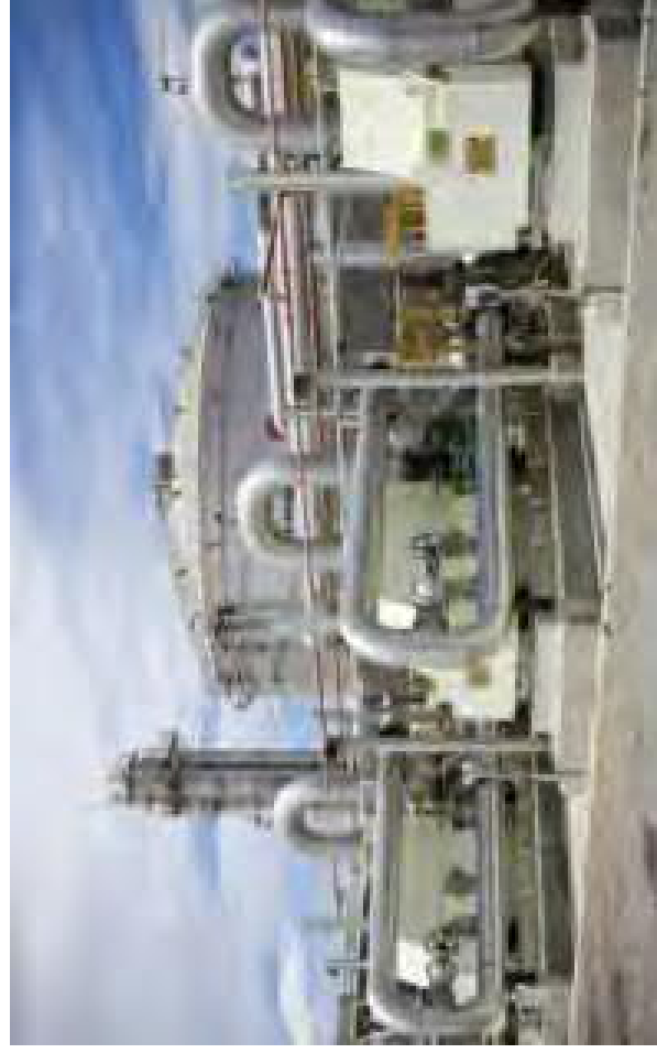
Example of a Central Processing Facility
