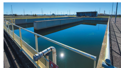
Collection basin for rainwater from the Bayet natural gas combined cycle power plant
