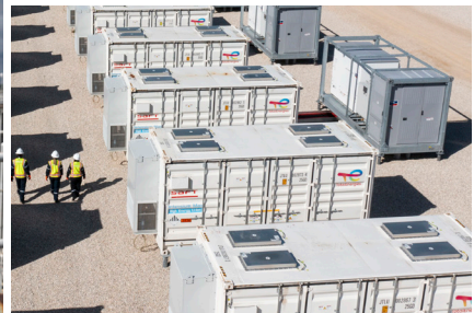
Battery-based energy storage systems at the Danish Fields solar farm in El Campo, TX.
