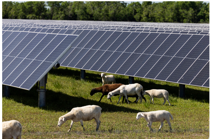
TotalEnergies focuses on sustainability at the Myrtle solar farm in Texas.
