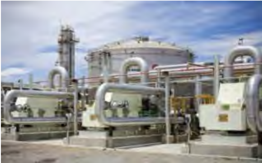
Example of a Central Processing Facility
